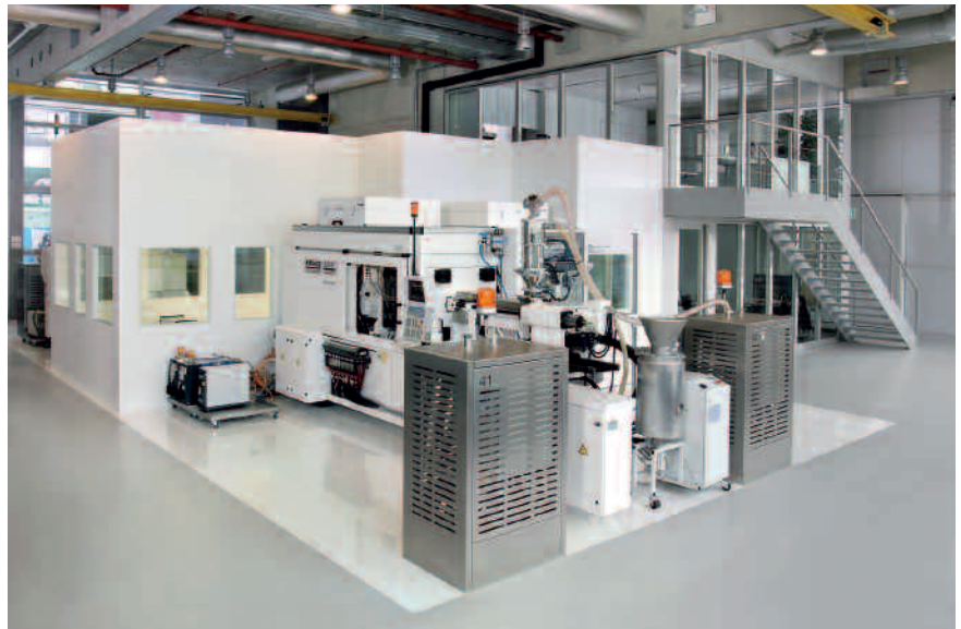
Fig. 4. High requirements in medical technology: The entire volume of air in the clean room is exchanged completely 80 times per hour (photo: Gira)
